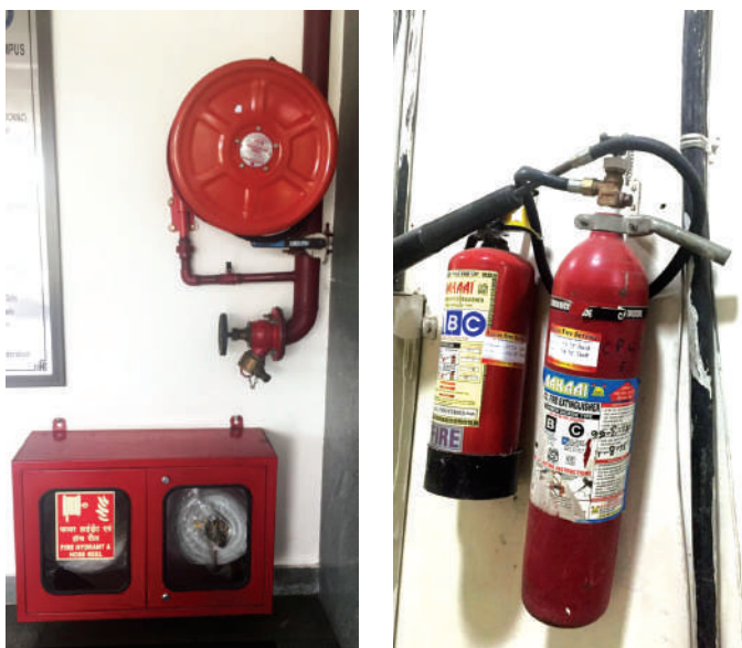
Fig. 5.1(a,b) Fire extinguishers
